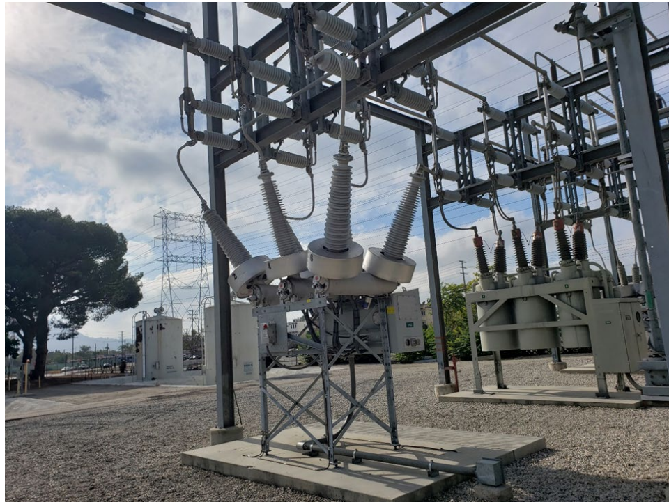
New Circuit Breaker Picture at RSE
