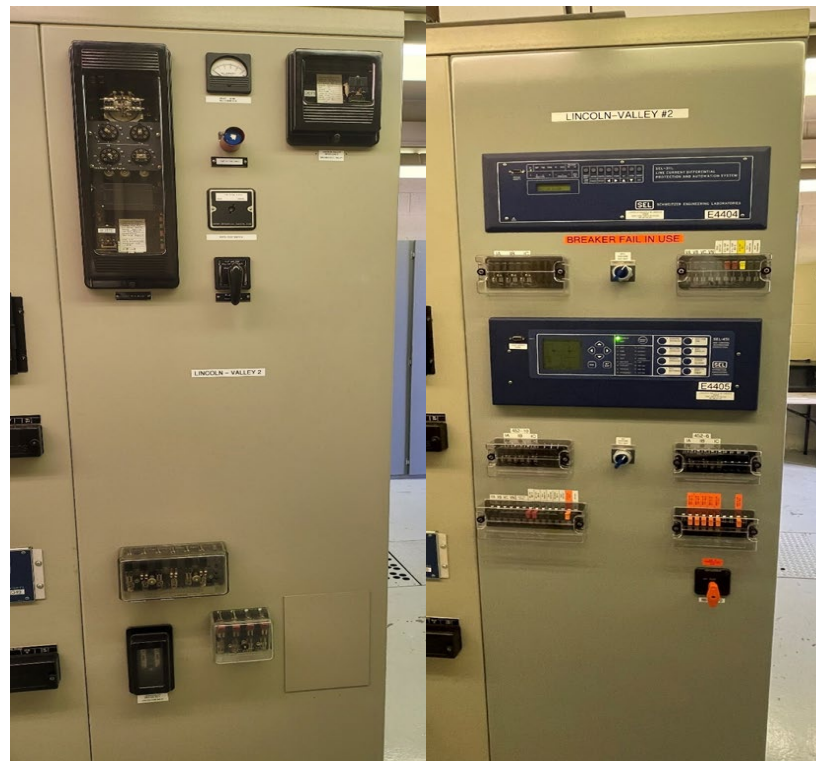
Old Relay Panel & New Relay Panel at Lincoln
