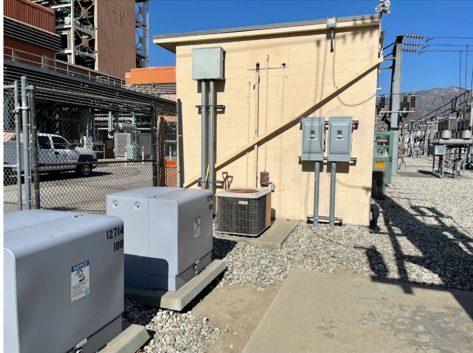
New Fused Disconnect Switch at Olive Sw. Substation
