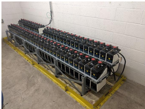
Battery Bank – Before Installation
