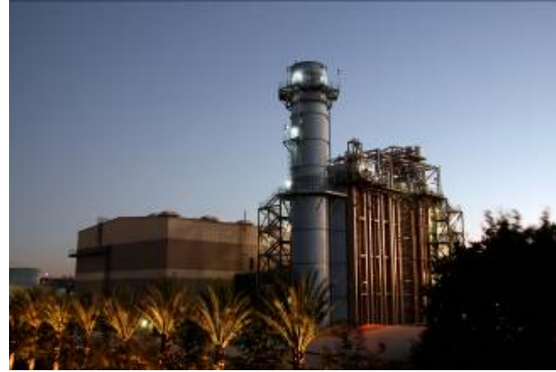
Magnolia Power Project
