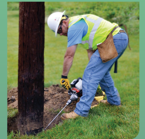
Worker inspects health of wooden utility pole
